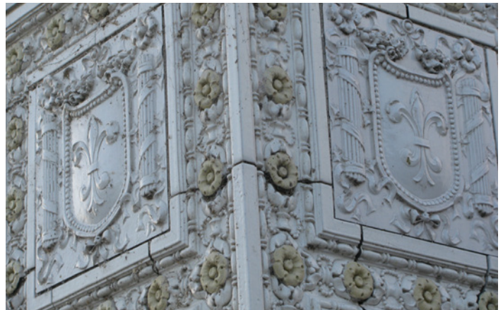
Architectural terra cotta is often highly decorative and a significant character-defining feature.
