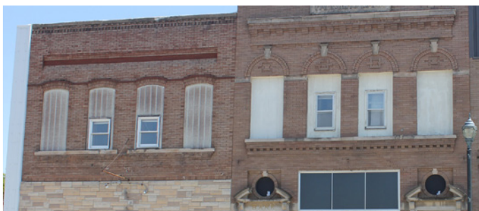
Infilled or reduced window openings are not appropriate.
