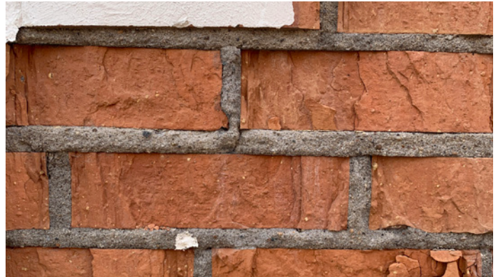
Mortar should be the sacrificial element in masonry; mortar that is too hard can cause damage to the bricks themselves.
