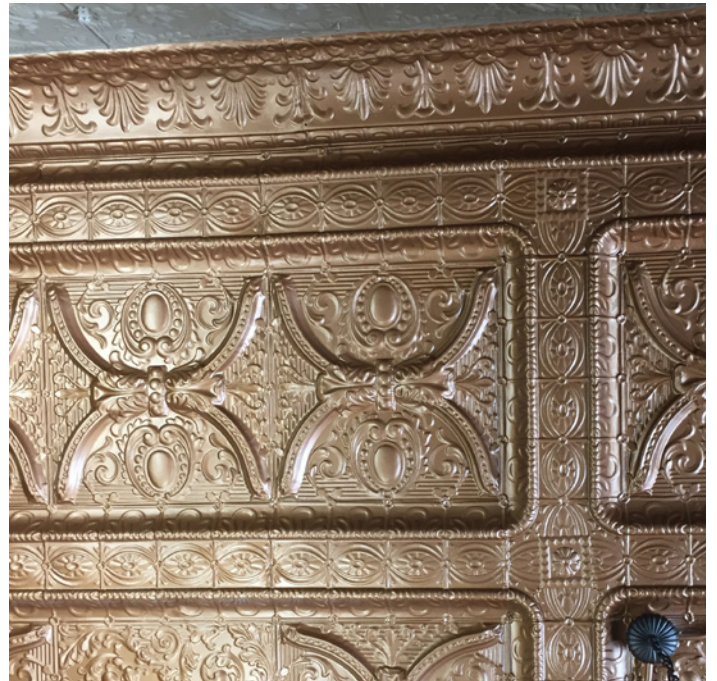
Restoration of historic tin ceilings can create a unique focal point for interior spaces.
