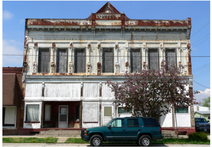
Paint failure and deferred maintenance has caused rusting and deterioration of character-defining features.
