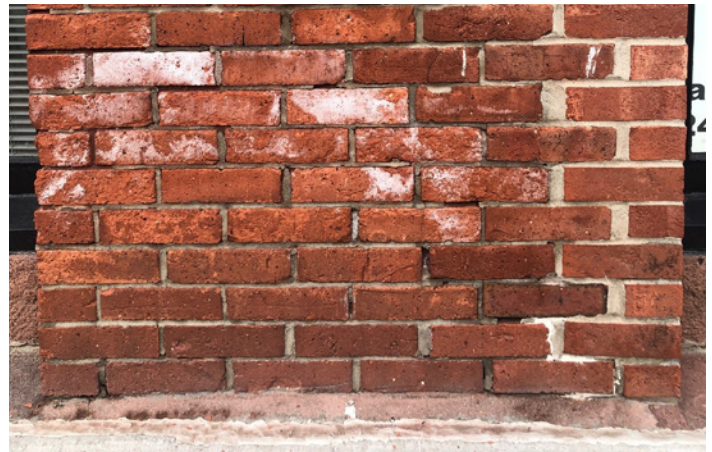
Poor condition of brick and mortar has led to water infiltration, causing material and structural damage.
