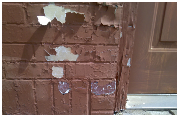
Peeling paint on masonry and wood can lead to deterioration of the underlying historic material.
