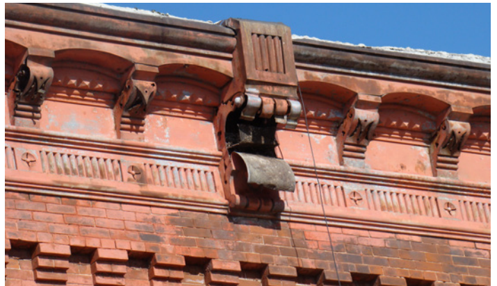
Metal cornices should be painted, and missing or damaged pieces should be repaired.
