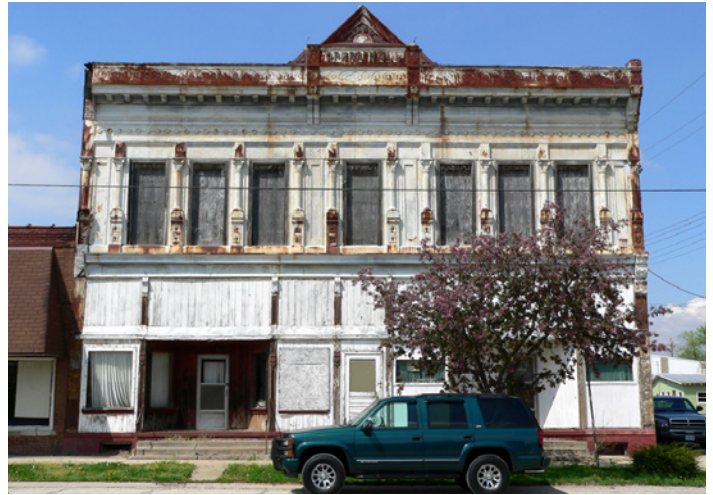
Paint failure and deferred maintenance has caused rusting and deterioration of character-defining features.
