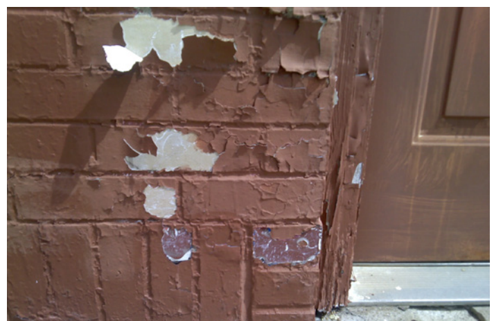
Peeling paint on masonry and wood can lead to deterioration of the underlying historic material.
