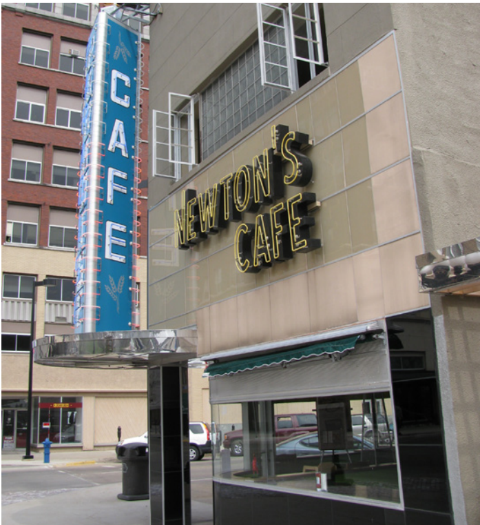
Structural glass panels and thin aluminum frames are character-defining features of this modern-style storefront.
