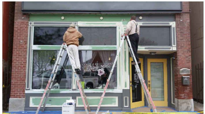
Restoring transom window openings is a key element in constructing a historically compatible storefront.
