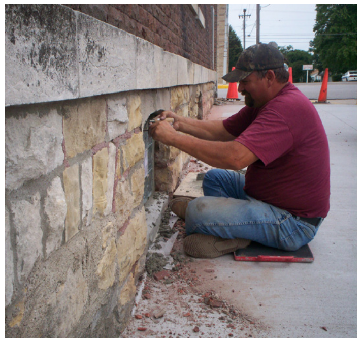
Mortar used for repointing should match original mortar in color, texture, and strength to protect historic masonry.
