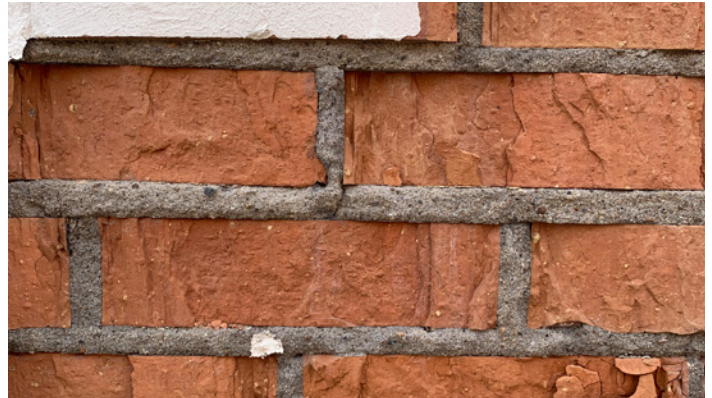
Mortar should be the sacrificial element in masonry; mortar that is too hard can cause damage to the bricks themselves.
