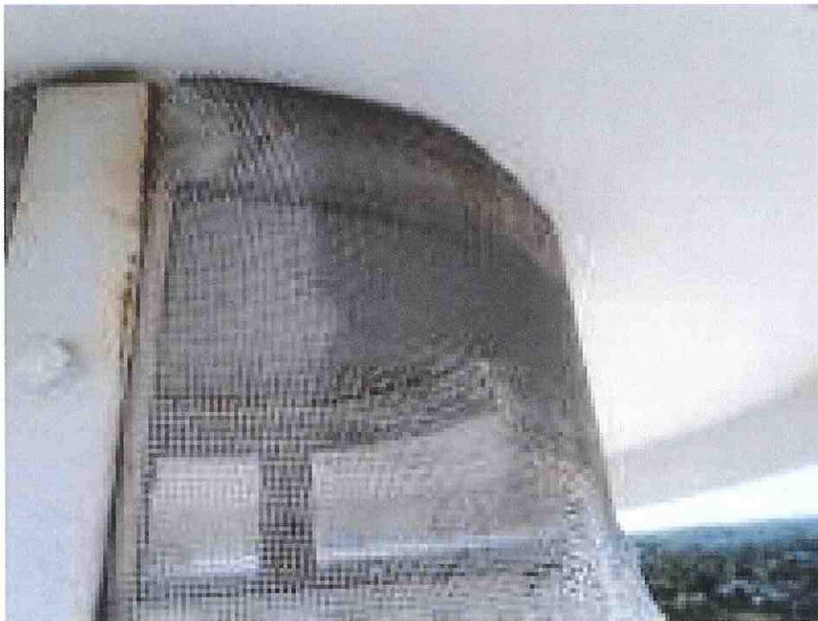
Replace with frost proof vent
