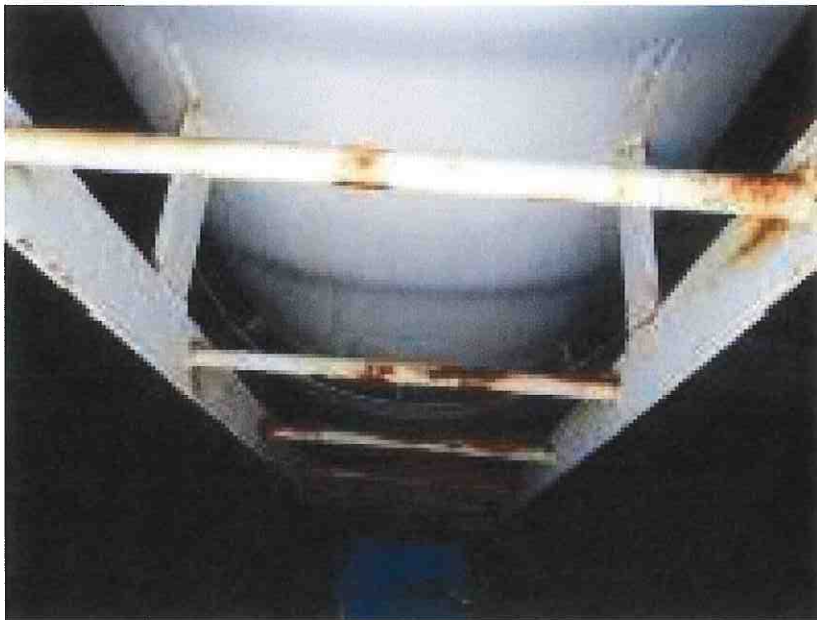
Replace top 5 feet of wet interior ladder
