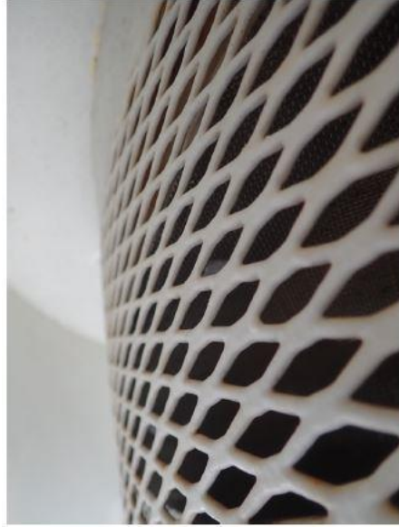
Vent screen to be replaced
