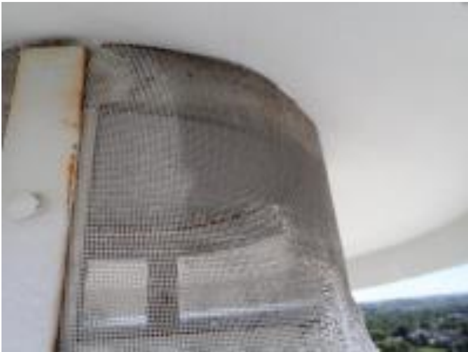
Replace with frost proof vent
